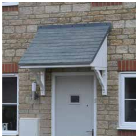
Unsuccessful example of plastic faux-tile porch, Banbury
