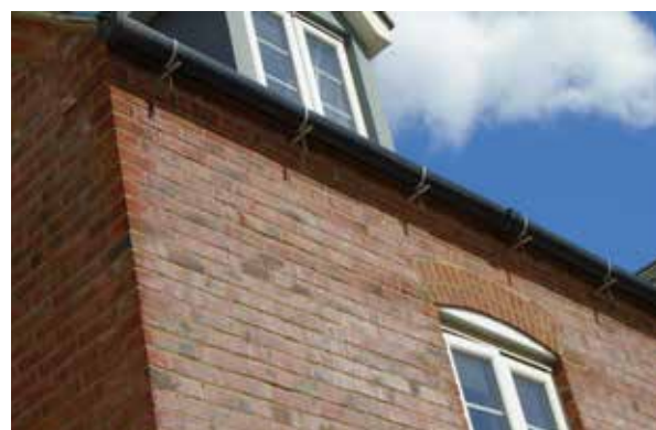
Guttering, South West Bicester
